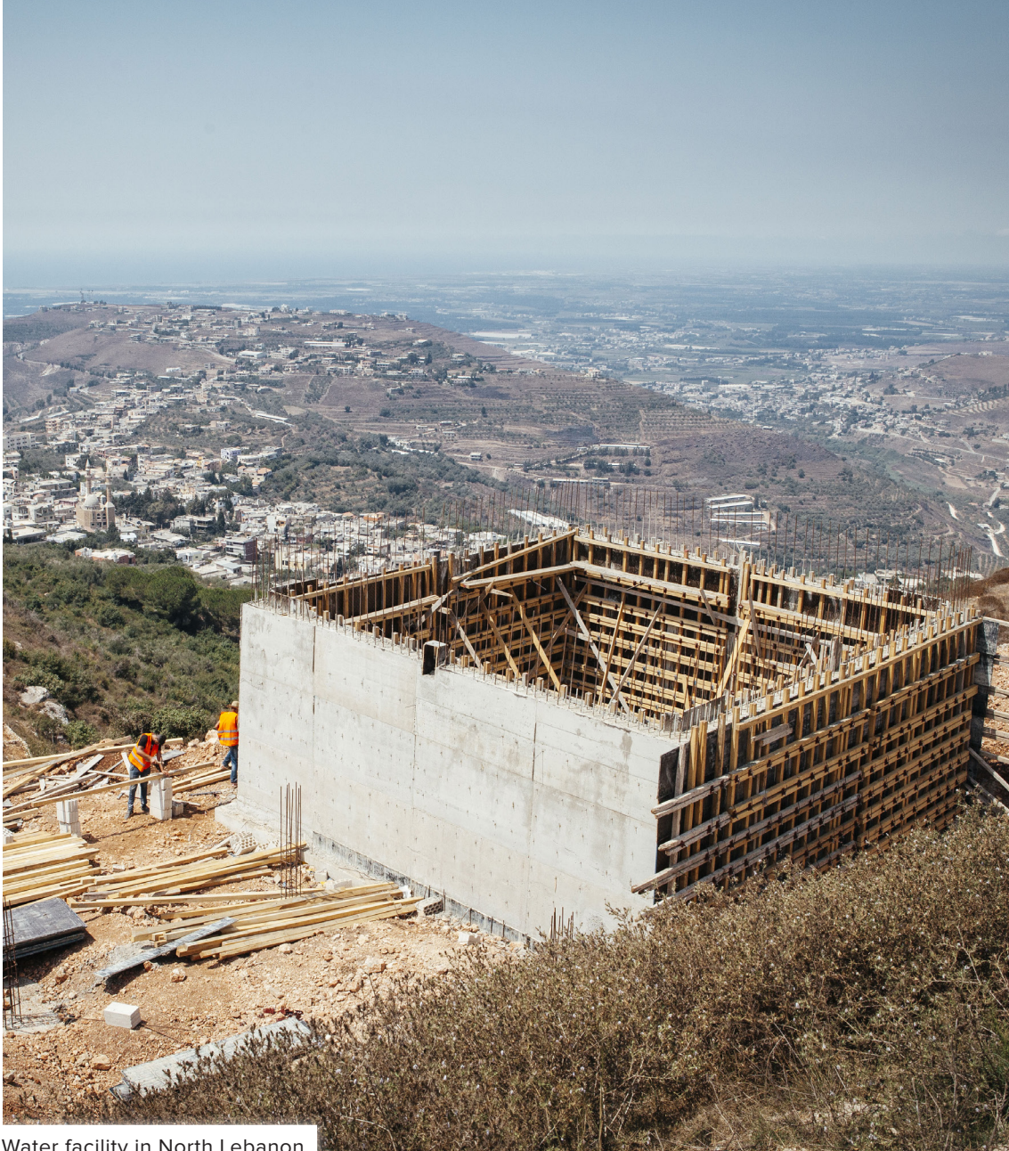
Water facility in North Lebanon
